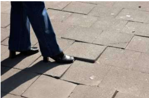
Pavements in a bad condition
